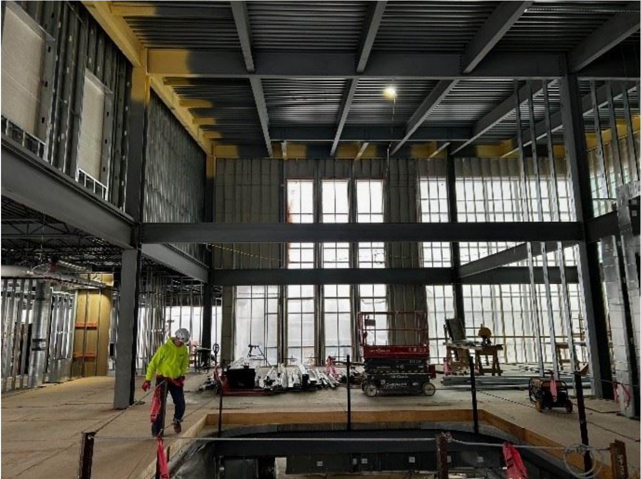
Figure 1 Staircase from the main entrance to the lower-level main entrance looking south
