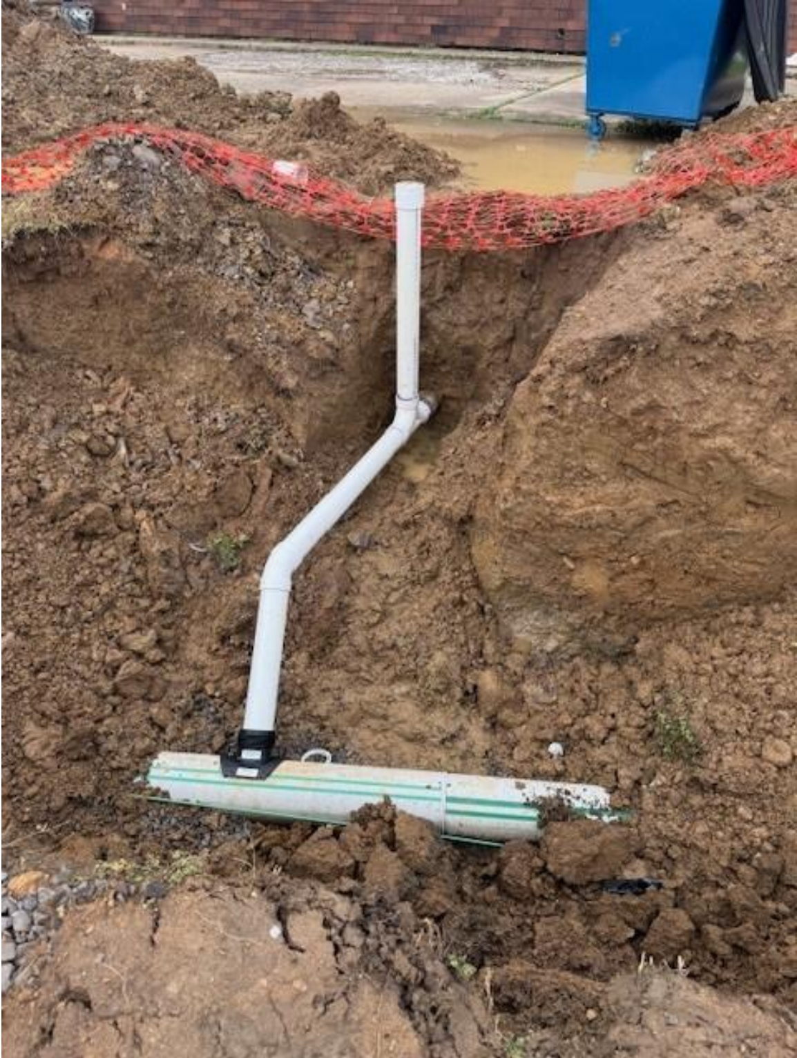
New 4-inch Sanitary Service and Cleanout on HDPE Installed by Pipe Burst
