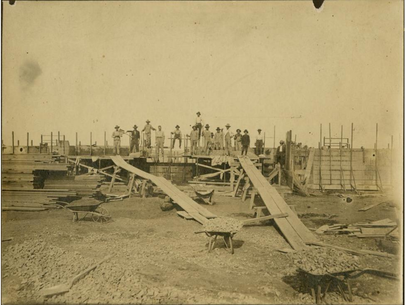
Figure 6. Photograph of Ferguson Hall under construction. Source: Hardin-Simmons University Library, The Portal to Texas History .
