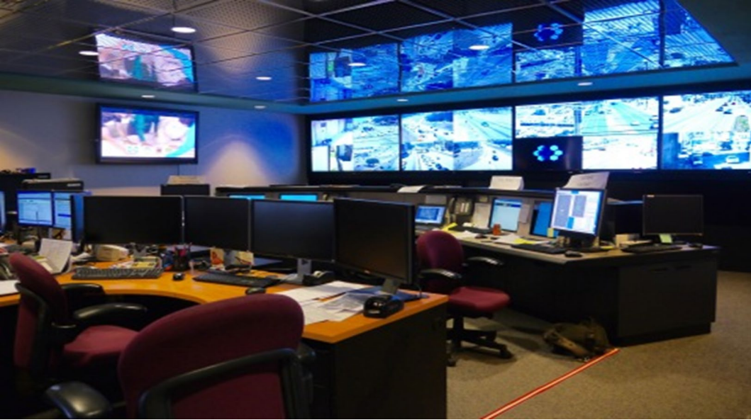
ITS Technologies, Traffic Management Center
