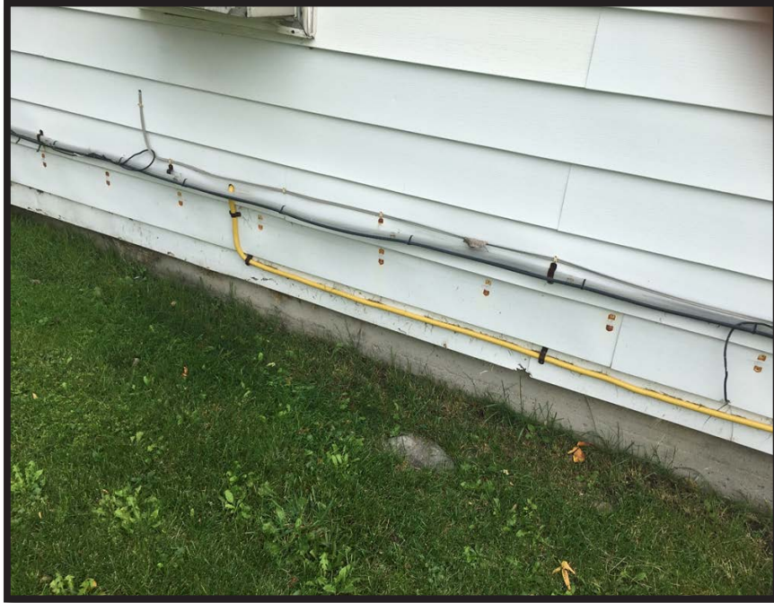
Flexible gas line used in an unprotected area (Relax Inn Motel, Watertown, Jefferson County DSS)
