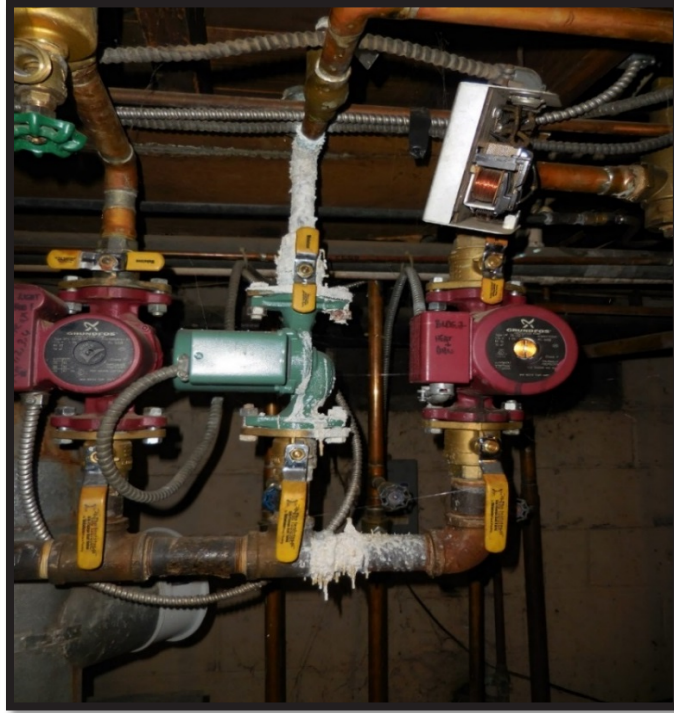
Corrosive build-up on boiler pipes (Budget Inn, Malta, Saratoga County DSS)
