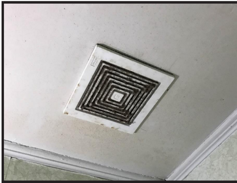
Mold on exhaust fan (Liberty Motel, Liberty, Sullivan County DSS)
