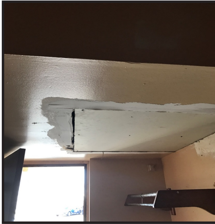
Water damage to ceiling in room with improper repair (Plantation Motel, Island Park, Nassau County DSS)
