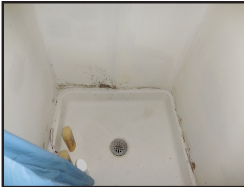
Mold in shower stall (Gateway Motel, Saratoga, Saratoga County DSS)
