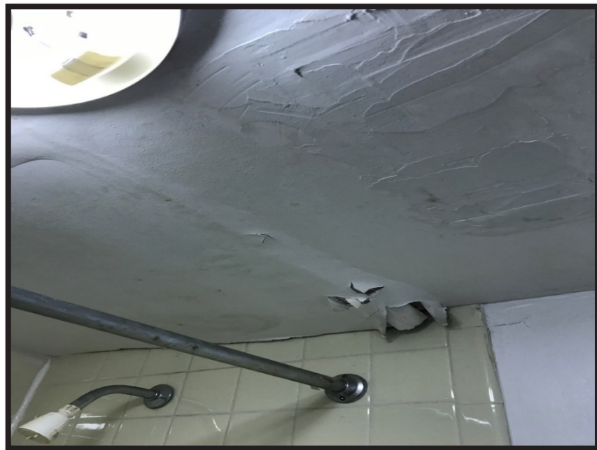
Water-damaged ceiling (Schuyler Inn, Menands, Albany County DSS)
