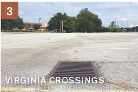
3 VIRGINIA CROSSINGS South of I-85, the creek appears in a stand of trees before it is capped beneath a 7-acre parking lot. Look down this storm drain to see the water rushing below.
